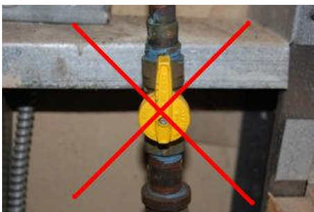
(Incorrect – Shutoff Valve is in the ON position)
