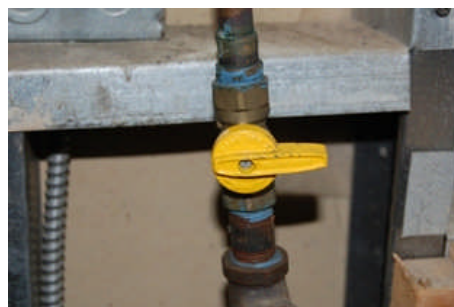
(Correct – Shutoff Valve is in the off position)
